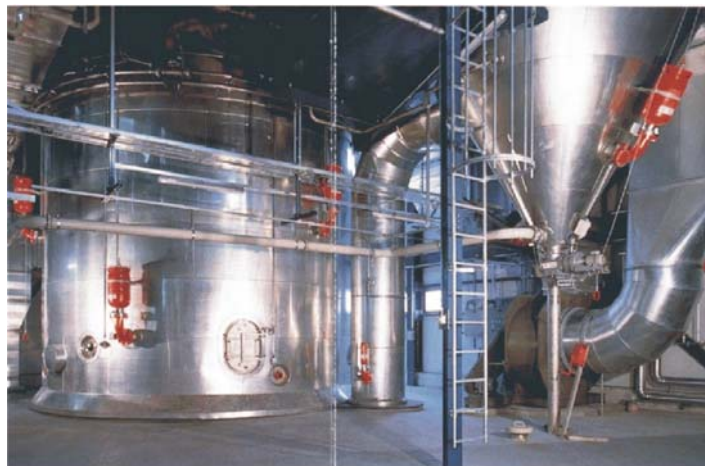
fig 3 pressure buffer tanks for suppression agent installed on the wall of a dryer
